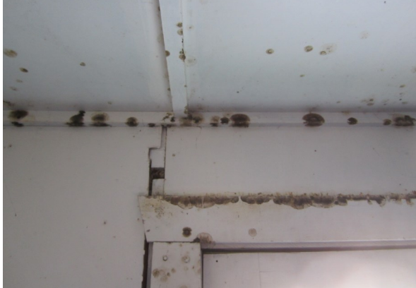
PHOTOGRAPH NO. 18 Mold on ceiling and door frame in main maintenance building.
