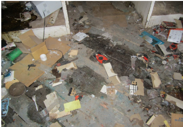
PHOTOGRAPH NO. 20 Stained flooring in the main maintenance building paint shop.
